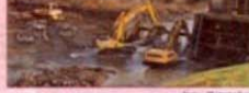
The old dam near Carbonton in Chatham County was removed in early 2006. The site had hosted several dams throughout the 19th century.
