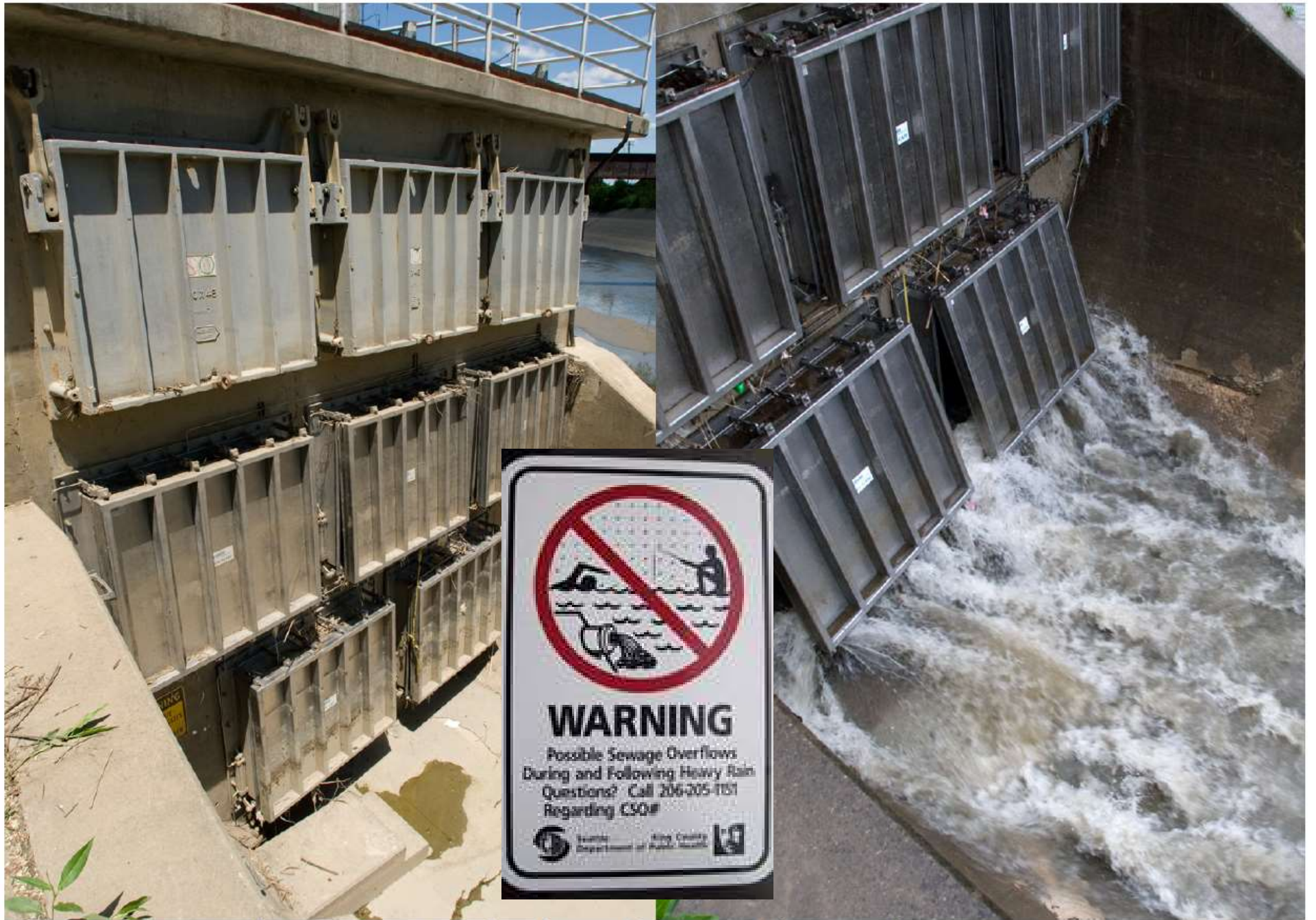
CSO #005 in South Fairmount under dry and wet weather conditions.
