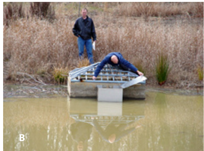
Figure 8. Downturned pipe on an orifice (A) and a trash rack in place around an orifice (B)
