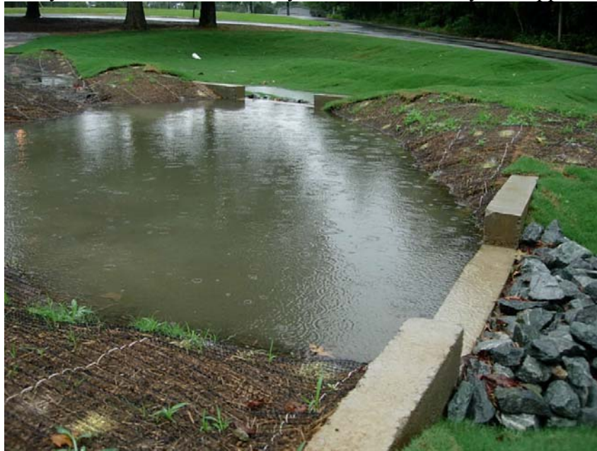
Figure 2. Forebay serving both of the bioretention cells. In the foreground (right) is one of the concrete weirs.
