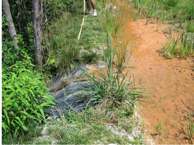
Figure 8: Breach on ABC stone level spreader
