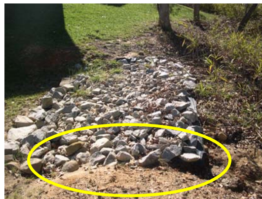
Figure 6: Rip rap level spreader with evidence of short circuiting
