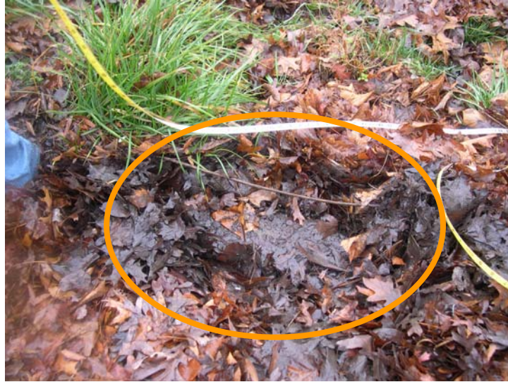
Figure 4: Level spreader lip buried beneath debris
