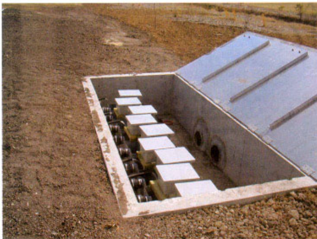
Figure 5. A concrete vault with flow gauges (enclosed in the boxes) and piping to samplers that collect water quality samples from the pavement surface runoff and subsurface exfiltrate
