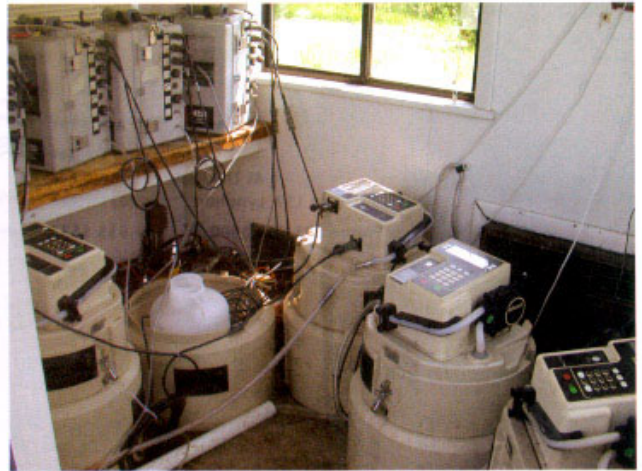
Figure 6. Flow meters and automatic samplers housed in a small shed collect runoff and subsurface exfiltrates from the pavements that drains to the adjacent concrete monitoring vault.
