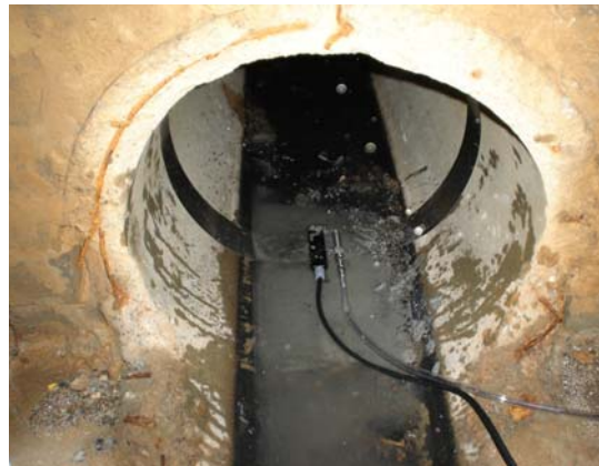
Figure 2: Sample area-velocity meter installation.
