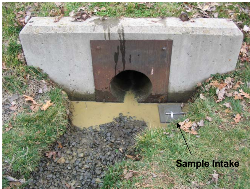
Figure 2: Outlet Monitoring at University Dry Detention Basin.
