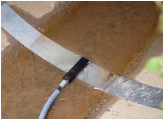
Figure 1: Area velocity meter installed in culvert
