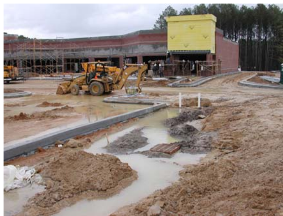
Figure 5. Sediment clogged the bioretention areas for long periods during the parking lot construction.
