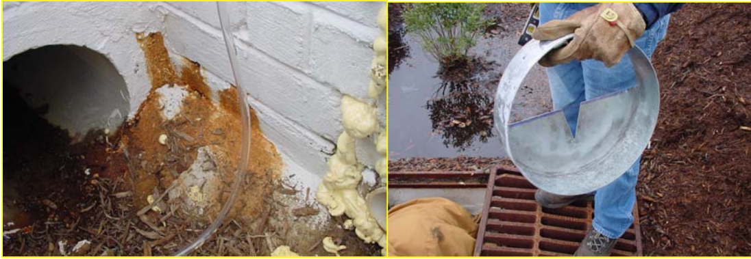
Figure 11. Each of the inlets leaked, as evidence in the picture in the left hand side of the figure. Flow sensors installed in an outlet would not capture all the flow leaving the bioretention cells. V-notch weirs, as shown on the right hand side were installed to measure flow leaving each of the cells.
