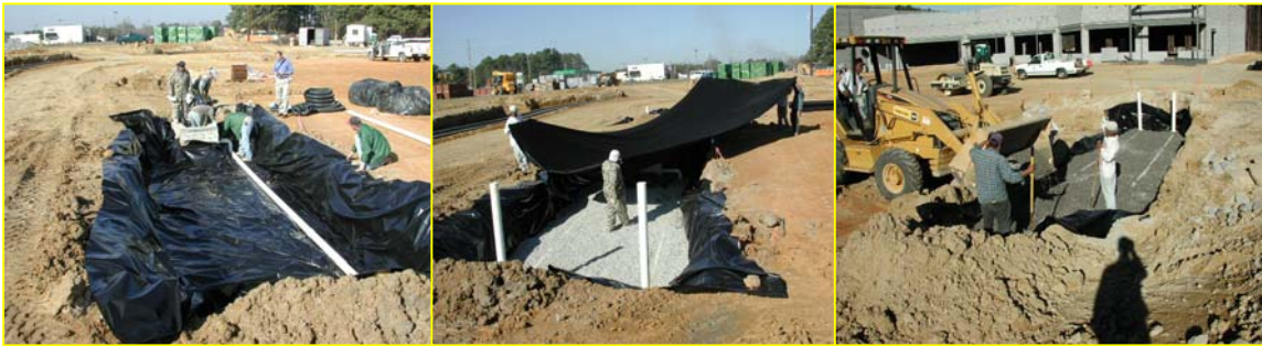
Figure 4. Bioretention construction in November and December in Wilson, NC. Pictured above are three phases from left to right: (1) installation of impermeable liner and drawdown pipes, (2) gravel drawdown layer with permeable geofabric about to be placed over it, and (3) fill soil being added to the device.
