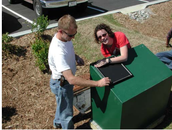
Figure 9. Monitoring equipment including automatic samplers was installed in Wilson during Summer 2002.
