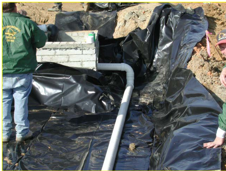
Figure 2. An upturned elbow in the underdrain pipe created an anaerobic zone in two of the four bioretention cells tested in Wilson.
