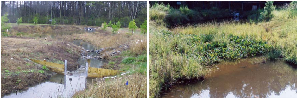
Figure 14. Stormwater Wetland at Wilson DOT CMY immediately after construction (left) and after two years of growth (right).
