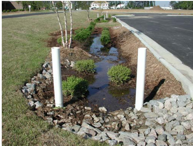
Figure 6. Four of the cells on the eastern side of the Wilson Parking lot pictured immediately after construction. These were the same bioretention cells pictured in Fig. 5.
