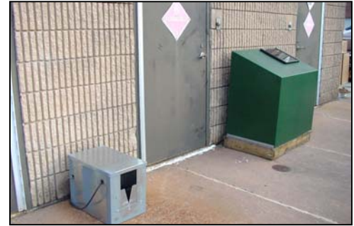
Figure 5. Sampling equipment for WCC control roof. Weir box is on left side; green sampler storage box is on right.
