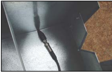
Figure 6. View inside the weir box with baffle, pressure transducer, and weir plate.
